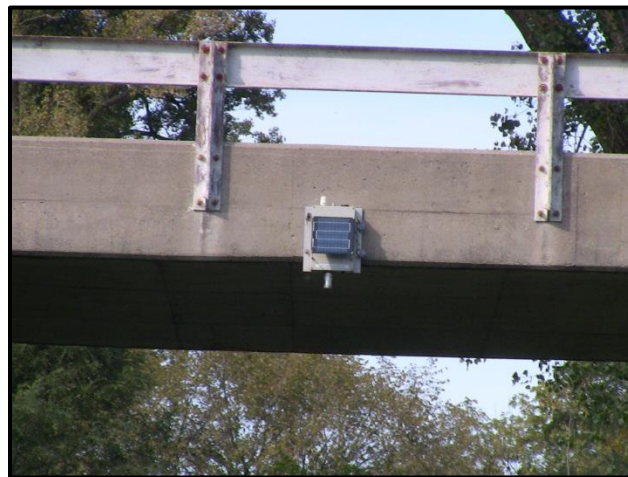
Figure 3.6: Iowa Flood Center stage sensor
